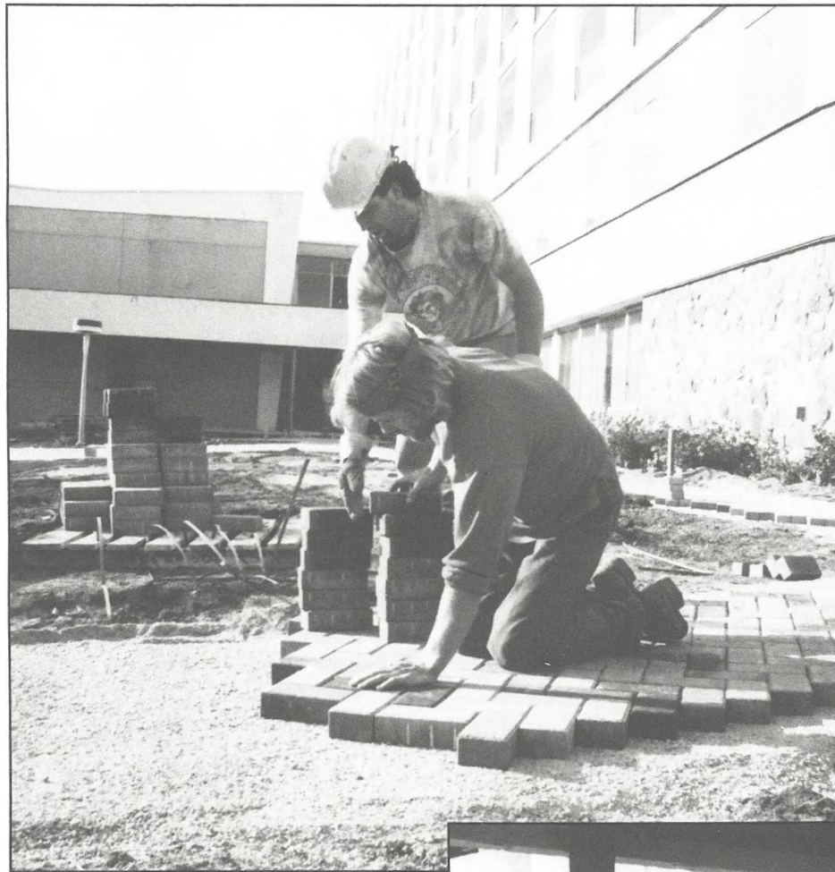
Workers laying the brick walkways in the courtyard. The landscaping has been donated by friends of OBC/OTS.
